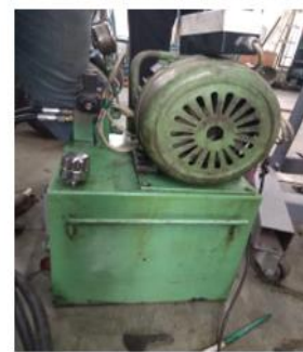
d. AC motor to drive hydraulic pump
