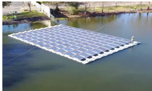
Figure 9 Floating Solar Plant
