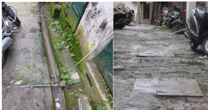
Figure 6. The existing sewer line in ward-4 Figure 7. Manholes at every 5m in ward number 4
