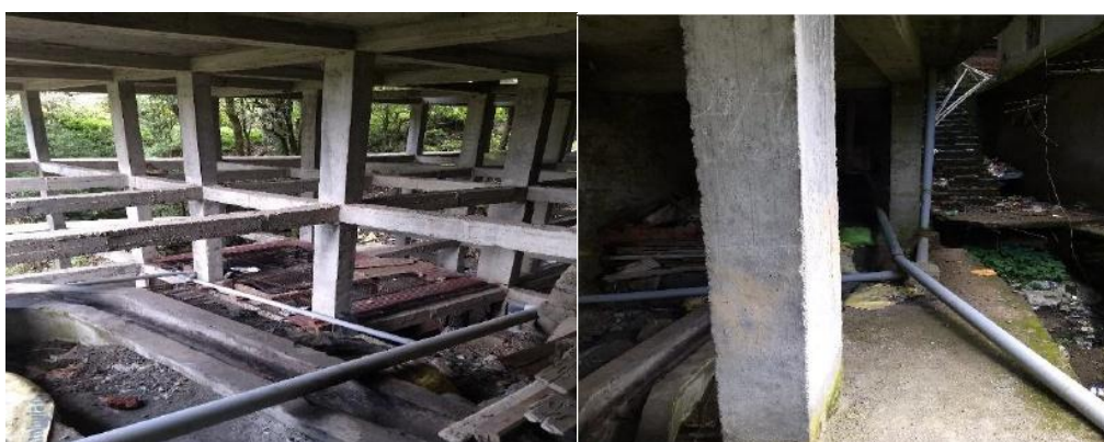
Figure 24. Proper containment and disposal of sewerage at Ravi Hotel of Ward-4
